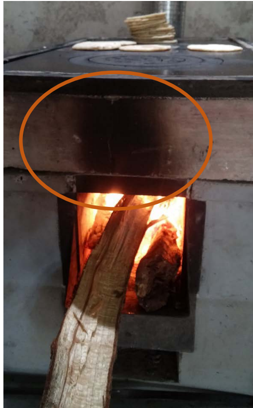
Figure 7. Evidence of back-drafting due to insufficient draught
